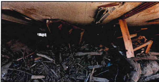
Debris caused by Hurricane Helene's floodwaters fills the fellowship hall to within inches of the ceiling at Pensacola UMC in Burnsville, N.C. (Photo: Mike DuBose, UM News)
