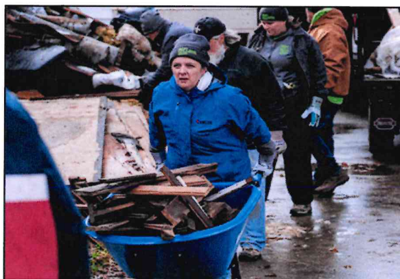
Katie Hills, UMCOR's director of Disaster Response, assesses the situation in Boone, NC, while pitching in with ERTs to clear debris from Valle Crucis UMC. (Photo: Ben Rogers, WNCC).
